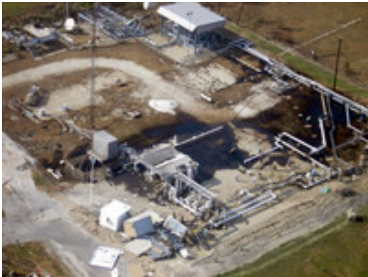
Chevron Pipeline at Empire Facility
